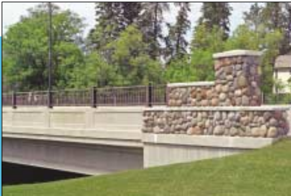
Part of the Edge of the Wilderness National Scenic Byway Corridor, this context-sensitive bridge reconstruction over Minnesota's Big Fork River applies rustic-style architectural and multimodal streetscape enhancements within the community. Photo Credit: Mn/DOT, Neil Kveberg.
